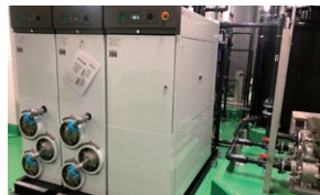
Water purifying equipment
