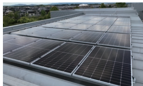
Solar power generation system
